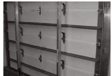
Reinforced Garage Door
